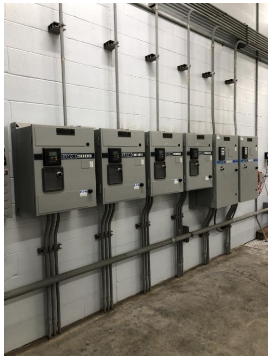
Treatment Plant Controls
