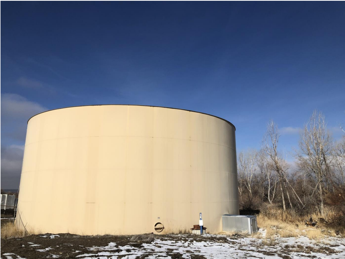
One Million Gallon Storage Tank
