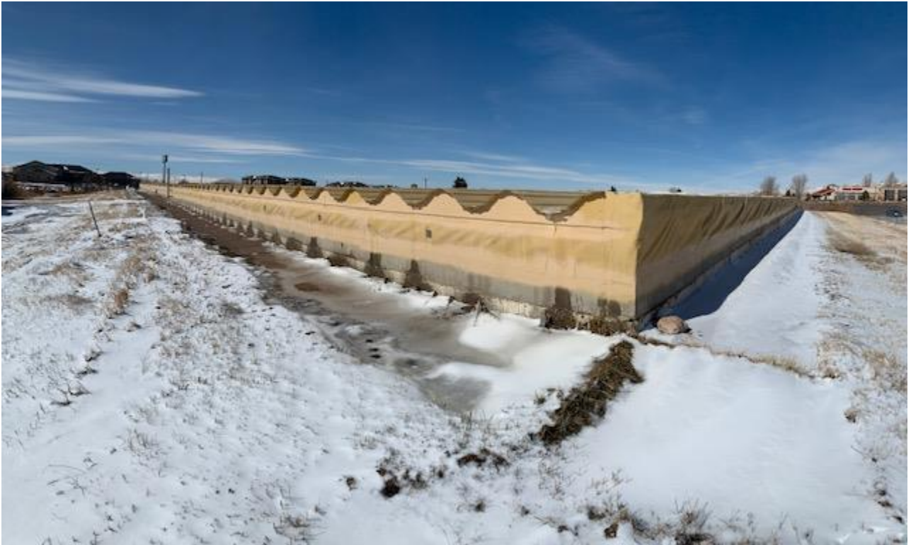
Zone 1 underground concrete water storage tank (8.5 million-gallon capacity) with significantly aging infrastructure concerns.
