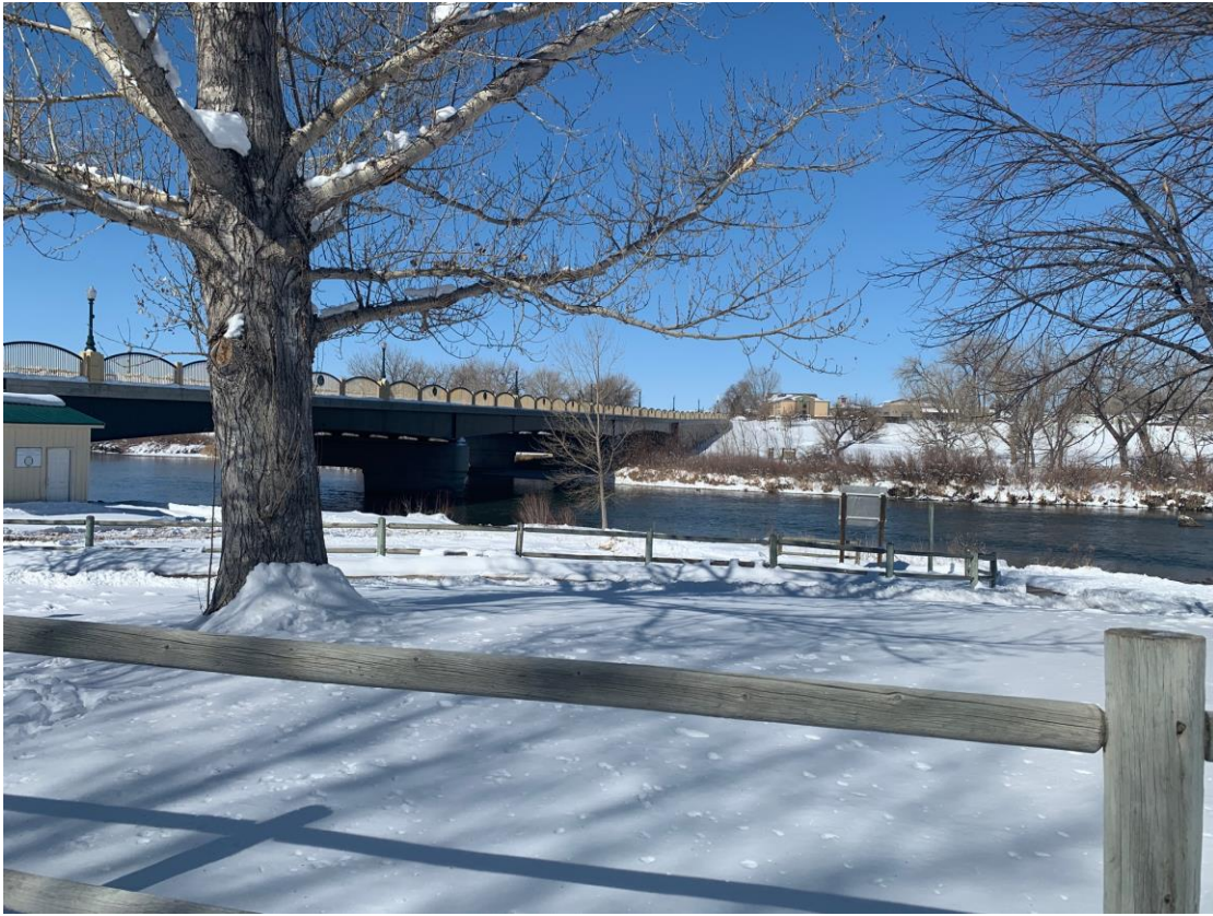
One of the two river water main line crossings on the North Platte River, west side of the City of Douglas.
