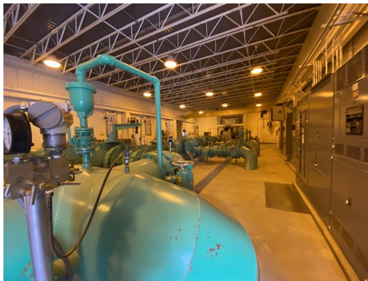
Booster Pump Station
