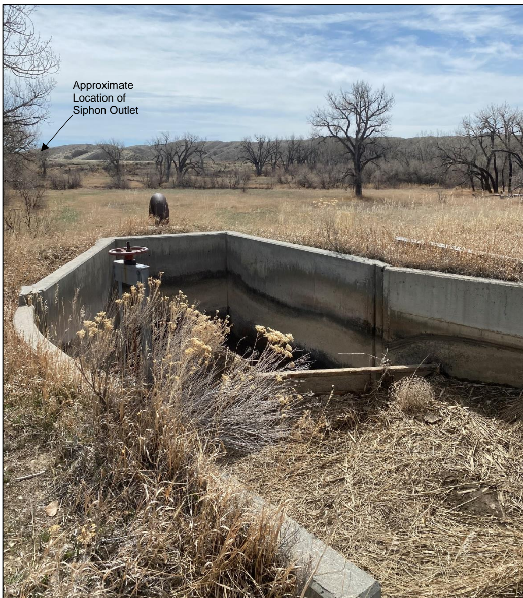
Siphon extending canal under South Fork Powder River was also constructed in 1994 and is reported to be in good condition. The Sussex Irrigation Canal has four siphons.
