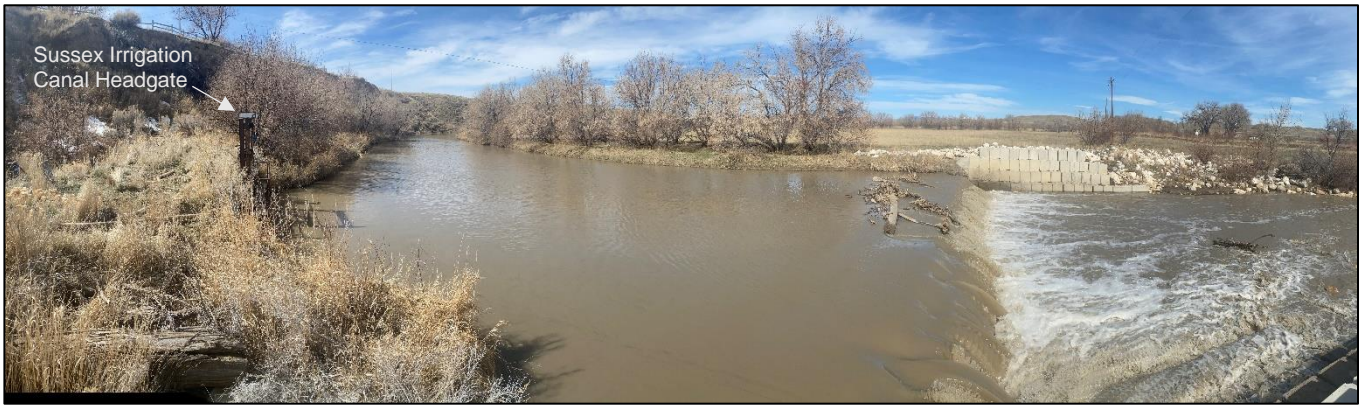
Middle Fork Powder River diversion dam and headgate (left) to Sussex Irrigation Canal. These structures were constructed in 1994 and are reported by the District be in good condition.
