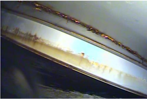
Roof and Support Beam Corrosion
