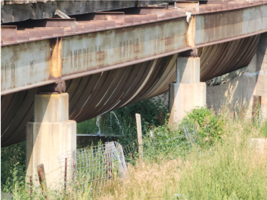
Leaks from the Flume Joints
