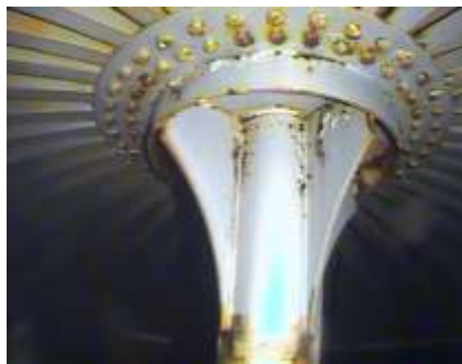
Center Support Column Corrosion
