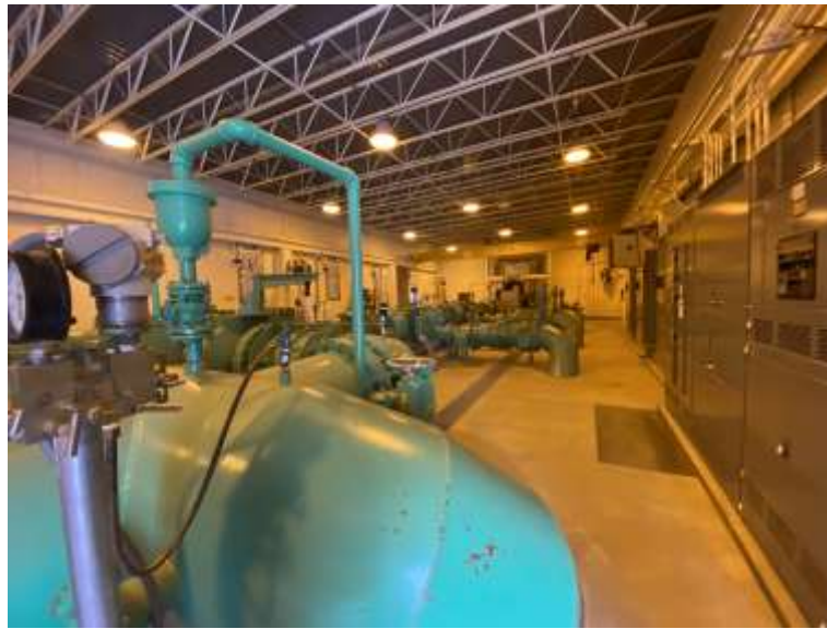
Booster Pump Station
