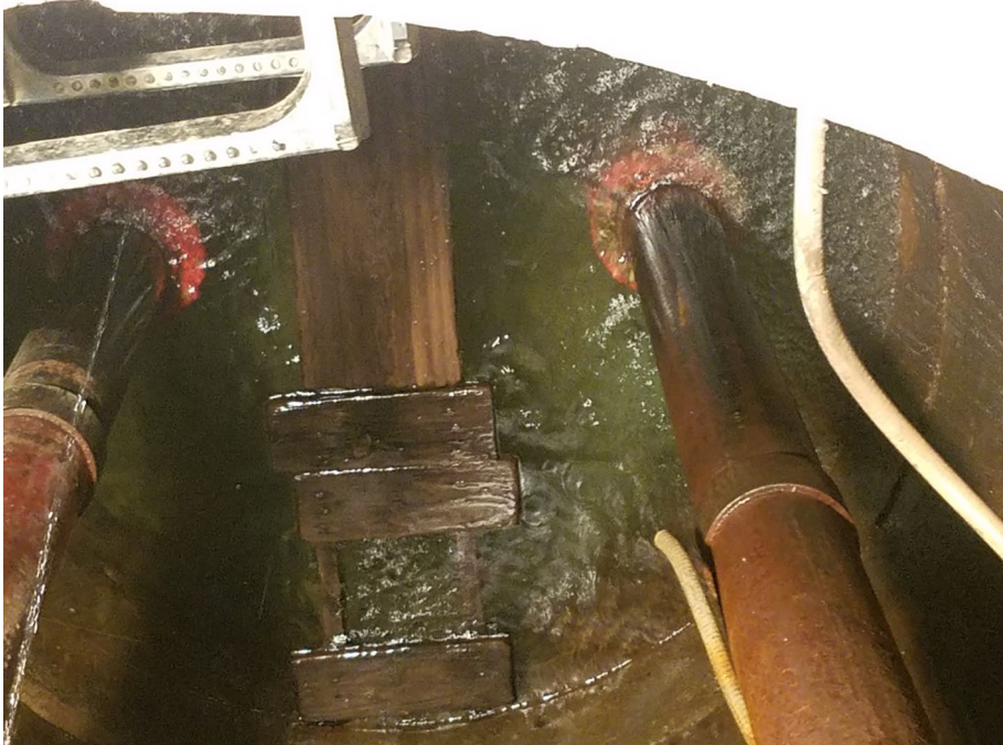
Infiltration Wet Well Pumps
