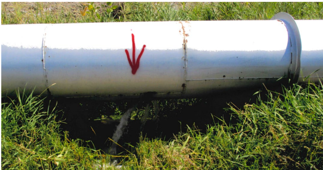
One of 30 Leaks in D56 Chute
