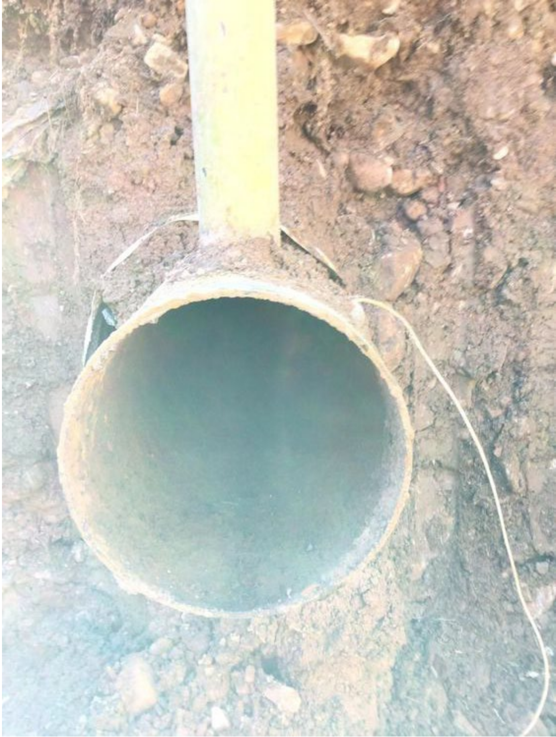
Example of pipe deterioration – Dry Creek
