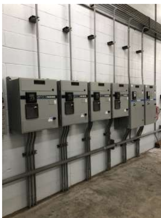
Treatment Plant Controls
