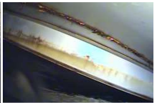
Roof and Support Beam Corrosion
