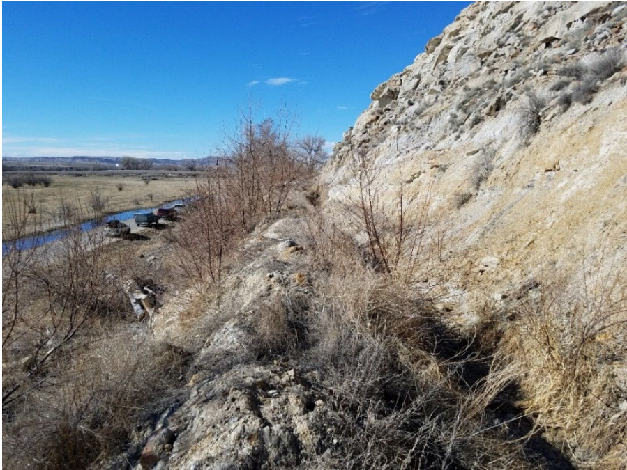
Kirby Ditch in slide prone area
