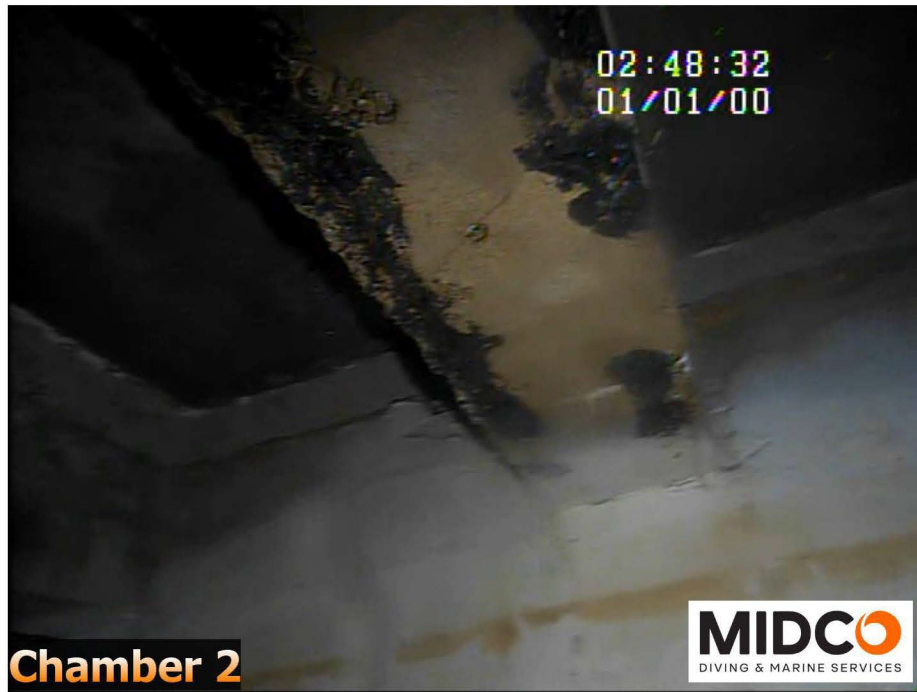
Typical Roof & Rafters – Spalling; Previous Repairs Noted
