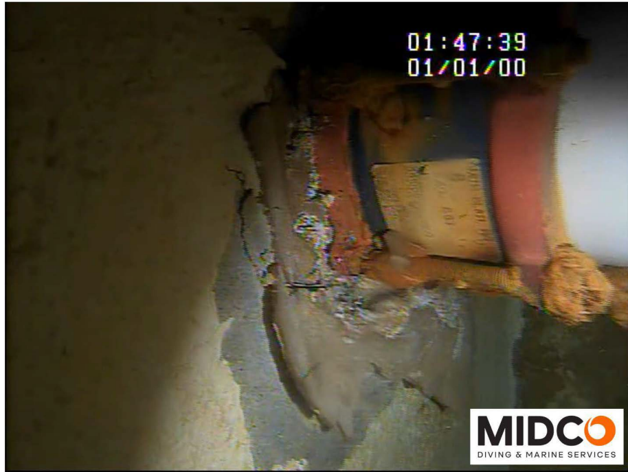
Inlet/Outlet #1 – Previous Repair Failure; Coating Failure with Corrosion Noted
