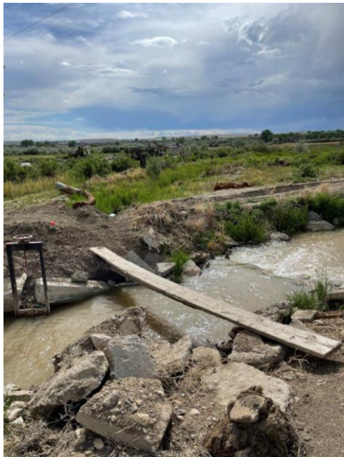
Tillard Canal Pump Station (top right) and Submersible Pumps (top left). Example of check structure (above).
