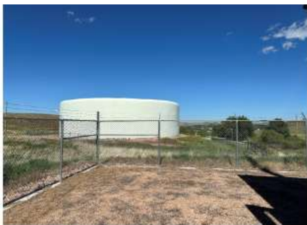
3 Million Gallon (3MG) Orpha Water Storage Tank, Douglas, WY.
