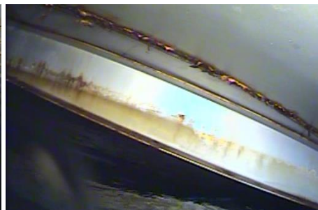
Roof and Support Beam Corrosion
