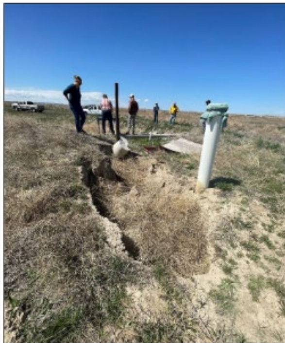
Sinkhole Above Malcolm Pipeline
