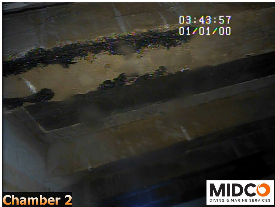
Typical Roof & Rafters – Spalling; Exposed Rebar; Previous Repairs Noted
