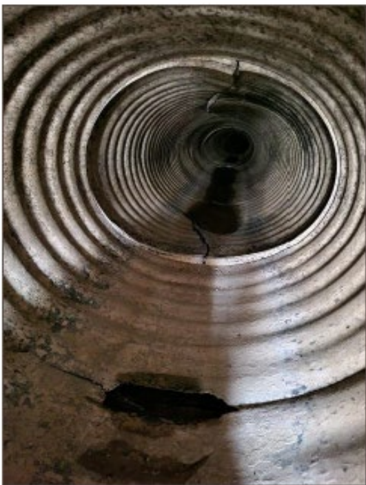
Malcolm Pipeline Deformation
