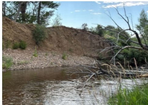
Unstable Section – Pioneer Canal
