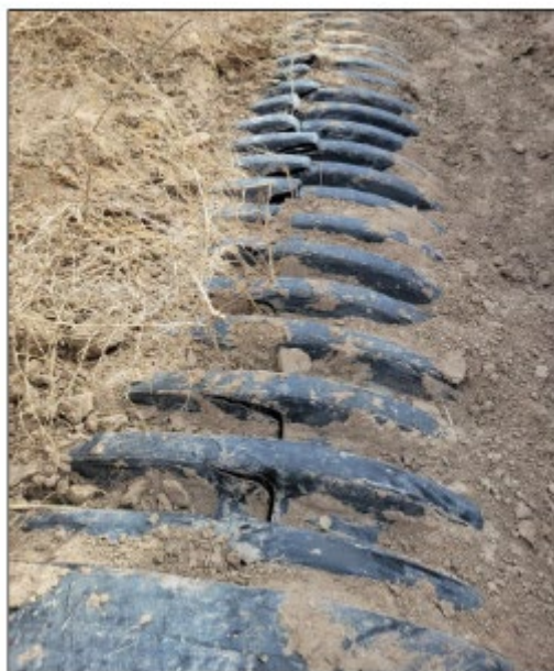
Exposed Fractures on the Malcolm Pipeline
