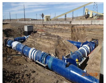
Source Water Supply Blending Facility
