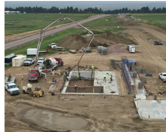
Sodium Hypochlorite Disinfection Facility
